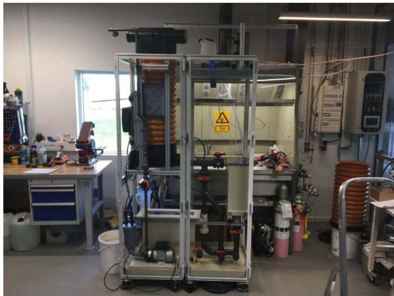
Slide 42 - Unit for electrocatalytic cleaning of biogas.
